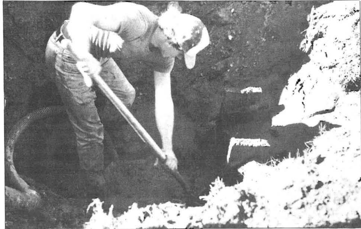
KNEE DEEP: A worker digs near Stadler Hall to uncover a broken water main Monday. The break caused sections outside of the Hall to be inundated with water before the main shutoff valve could be reached. The main campus was without water service for several hours until workers could repair the main.
