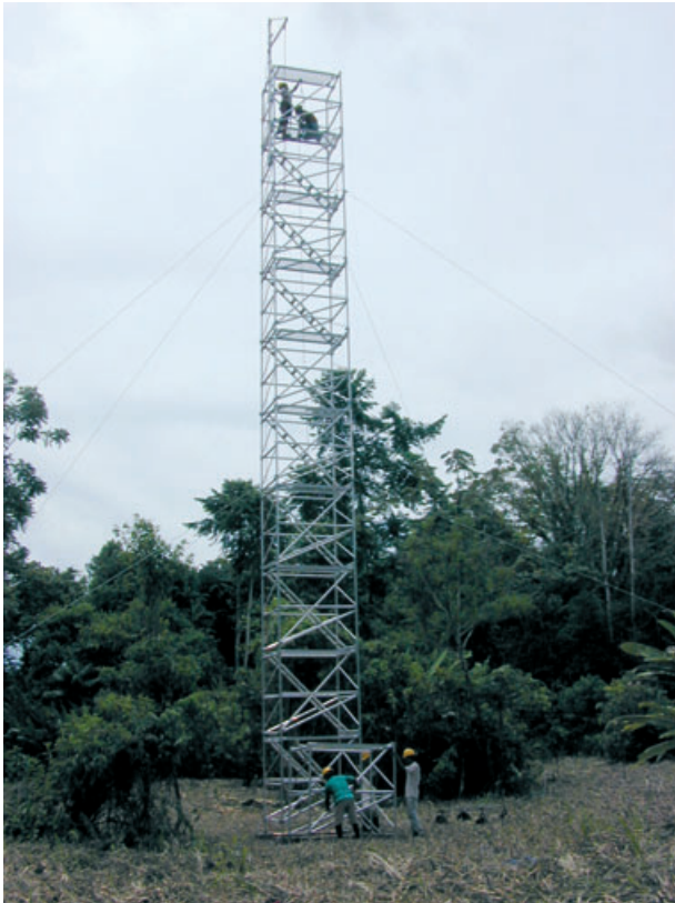
Figure 1 Construction of a practice tower in an open field. Tower is at level 10 (18.6 m tall) of 24 possible levels (sections). Field crew is preparing to lift another section using a small davit visible to the left of the top installed section of the tower.
