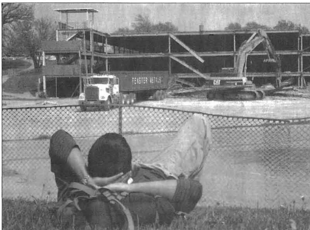
Goodbye, Garage D...Hello MSC Lakes. UM-St. Louis demolished the deteriorating Garage D, which had been around for over 25 years. A new parking lot and two new lakes took its place. The garage was taken down in April, 2004.
