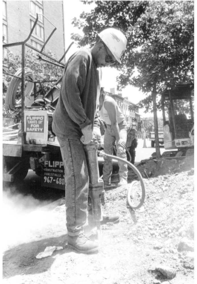
Air hammer operators use machines with interchangeable hammers to cut or break up old pavement.
