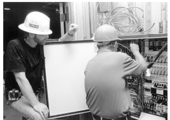
Elevator installers need a working knowledge of electricity, electronics, and hydraulics.
